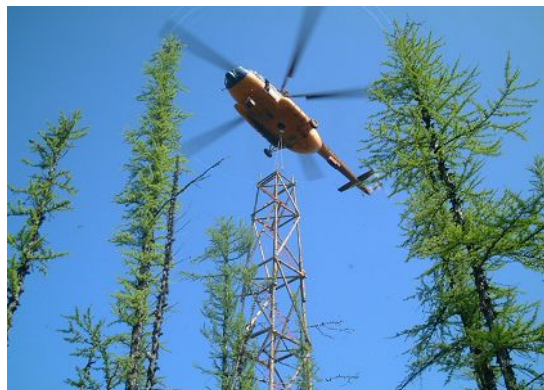
Fig.3 The helicopter, transporting the tower to the site (photo by Dr. Matsuura)
